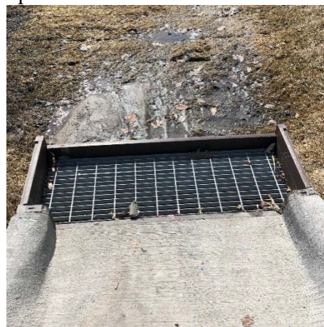
Rain Guardian in Need of Maintenance
