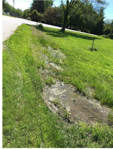
Grass Swale with Standing Water
