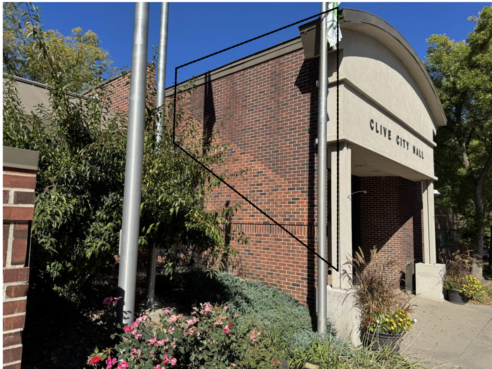
TYPICAL EXAMPLE OF BRICK STREAKING
