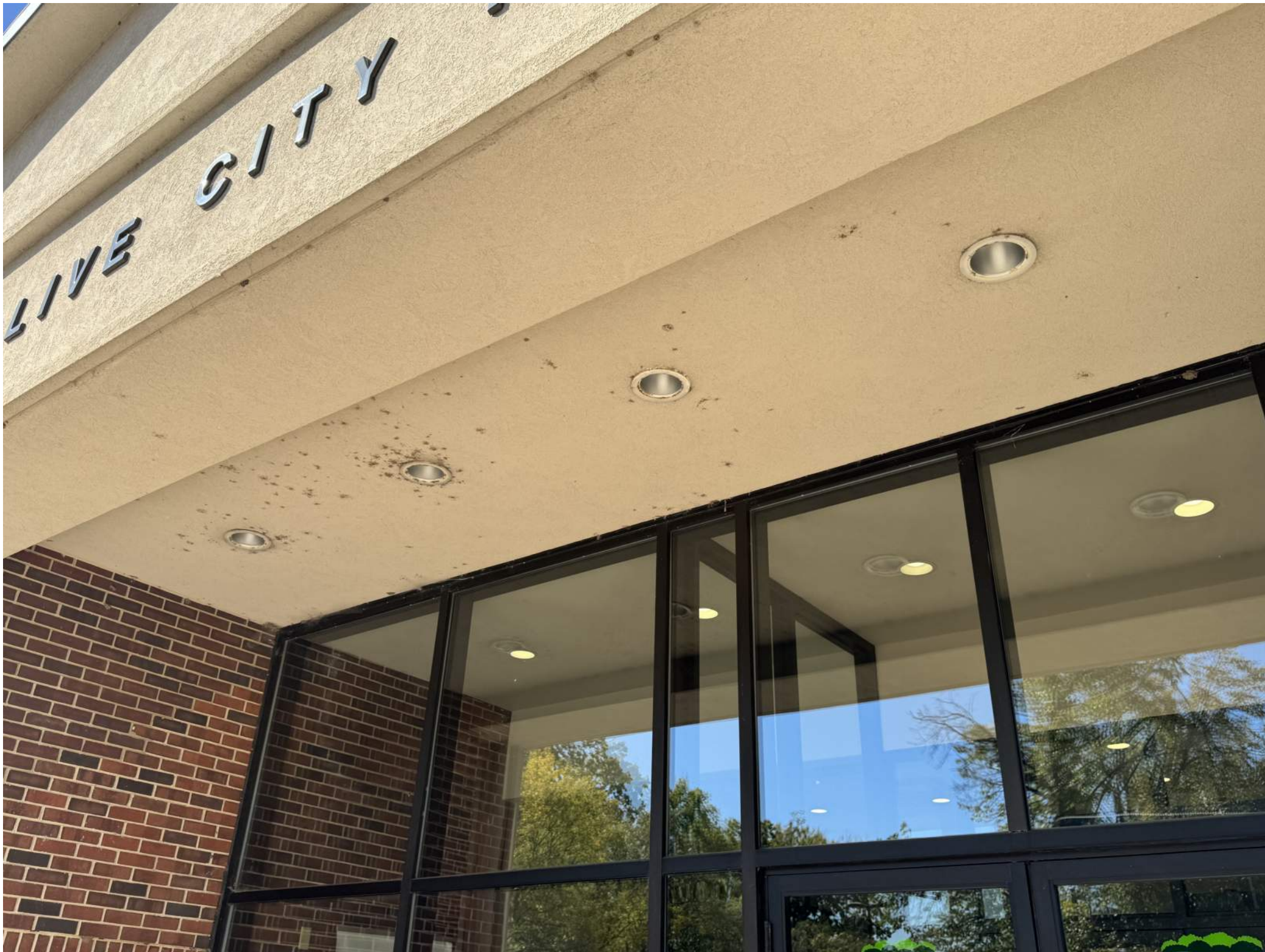
EXAMPLE OF DIRTY SOFFIT AT CITY HALL ENTRY
