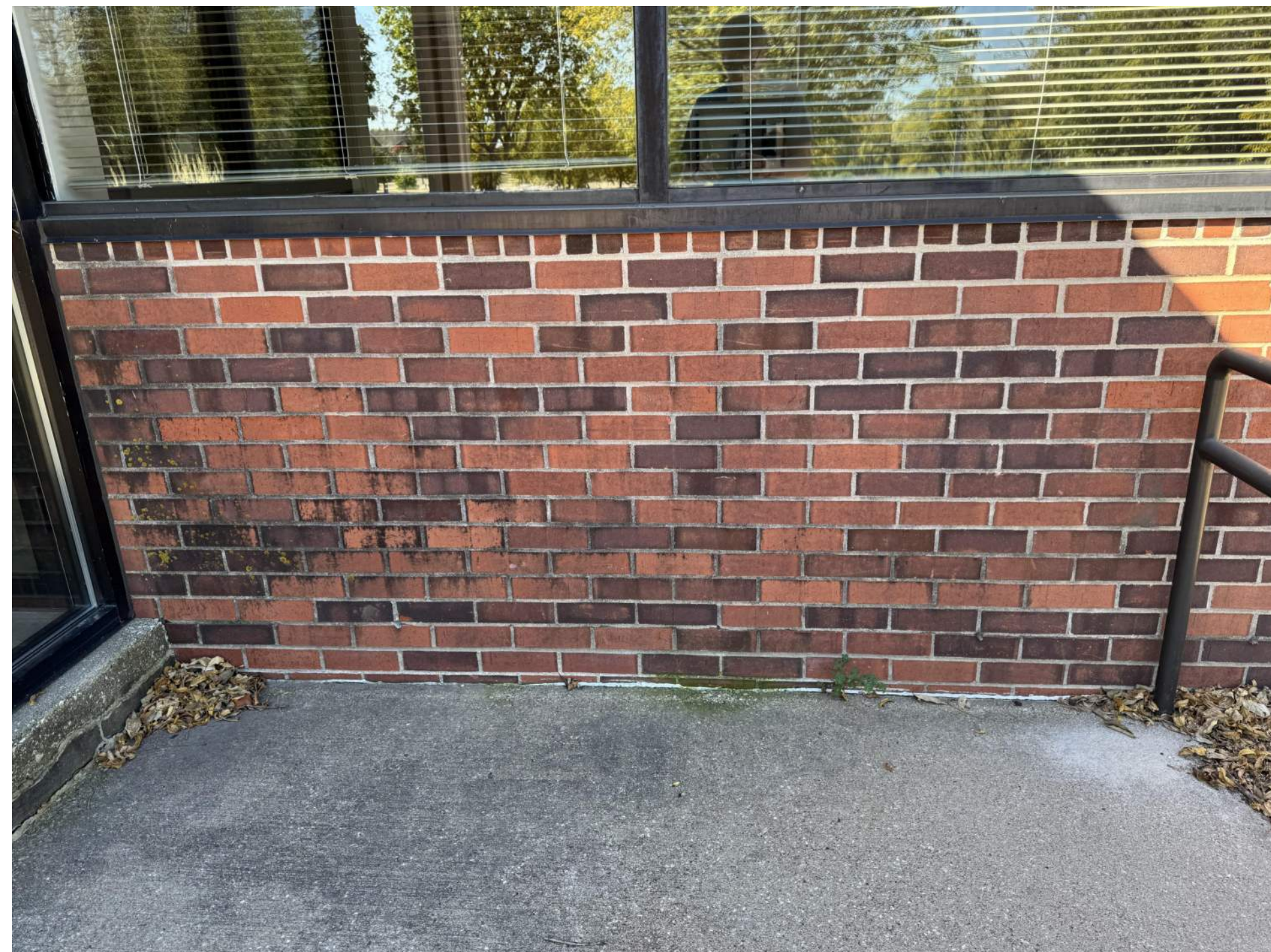
EXAMPLE OF DIRTY BRICK NEAR CHAMBERS ENTRY
