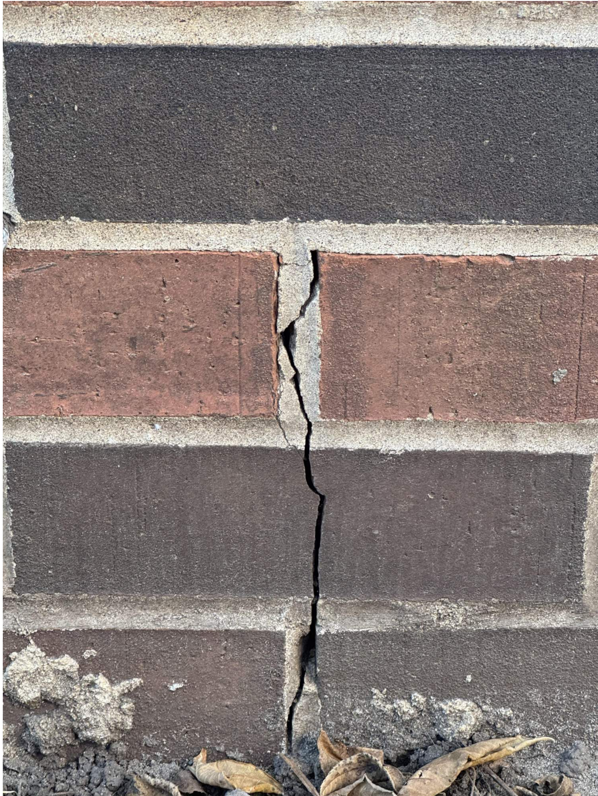
TYPICAL BRICK CRACK AT GRADE TYPICAL CRACKING TO BE REPAIRED AND SEALED
