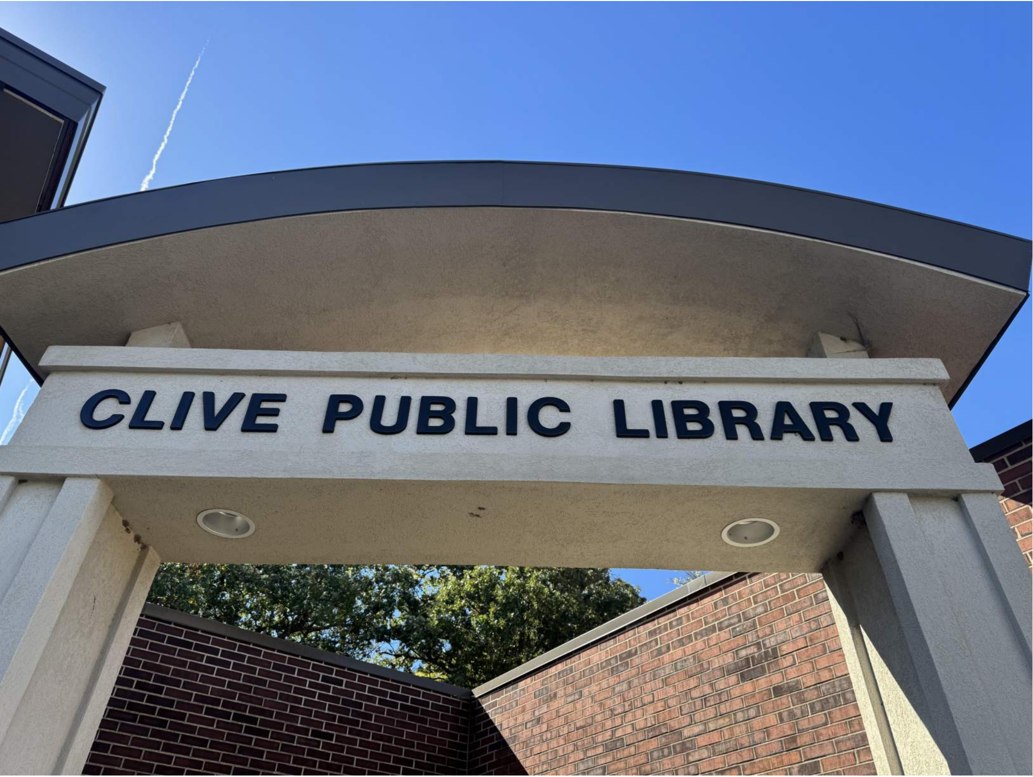
EXAMPLE OF DIRTY SIGNAGE AT LIBRARY ENTRY
