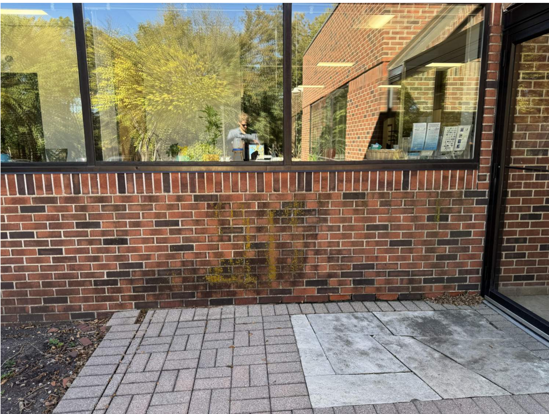
EXAMPLE OF DIRTY BRICK NEAR PEDESTRIAN PATHWAY
