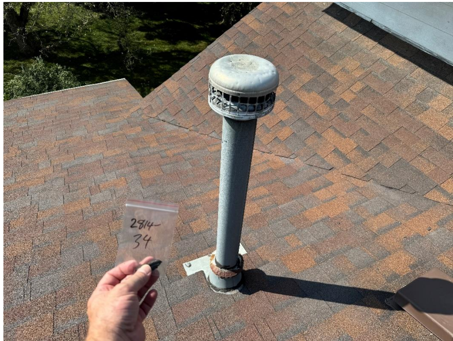
Representative View of the Asbestos Containing Roof Tar. (2814-39 {misabeled as 34}, 2% Chrysotile)
